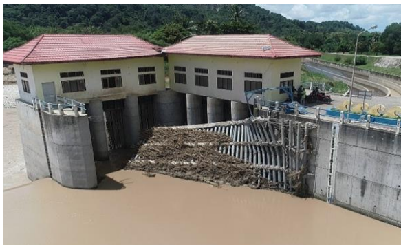
Trash Rack Bendung Benanain, Kab. Malaka
